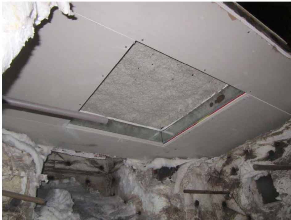
Exposed Side Prior to the Fire Test
